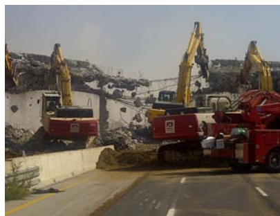
Left: Parkway crews work to remove the North Talbot Road Bridge over Highway 401.
